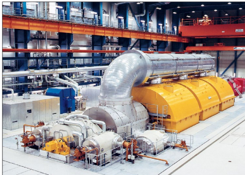
Typical production turbine used in large-scale power-plants. The project described called for each turbine to be secured individually.
