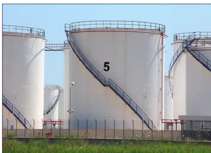
Oil storage tanks include a host of security measures, both physical and cyber. Each tank houses multiple sensors and controllers that control the environmental conditions inside the tank.
