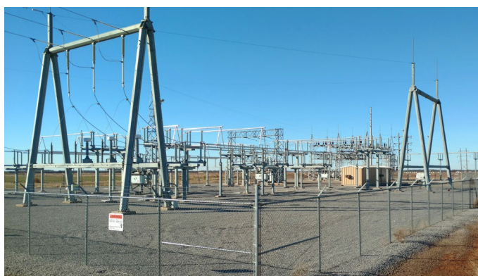
One of the Radiflow-equipped substations included in the project
